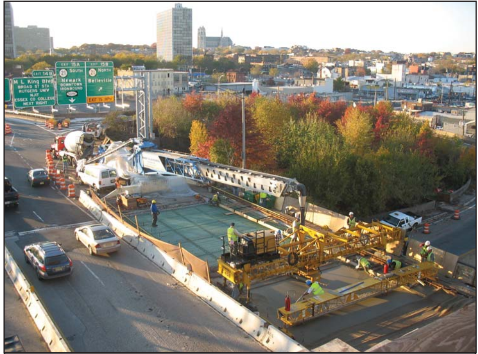
The placement of a light weight concrete mix on the Exodermic Deck system that was installed.
