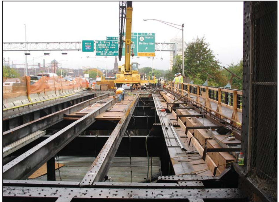
New structural steel members set in place for a portion of the Stickel Bridge rehabilitation.
